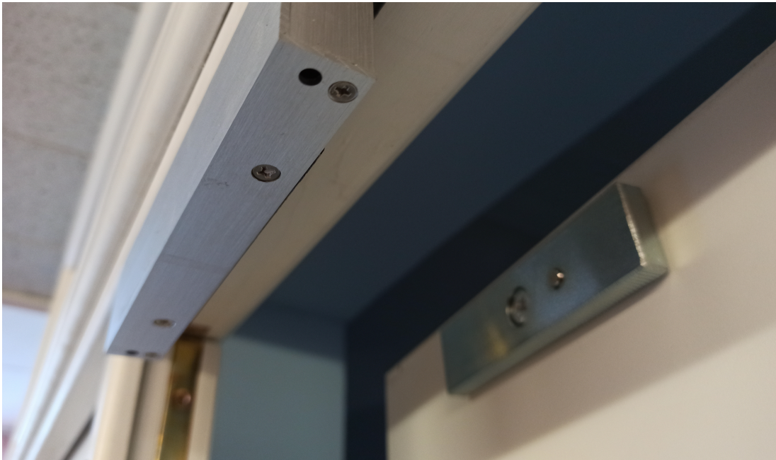
Figure 4: Electromagnetic locks mounted on a door. Source: AndreyKac/Shutterstock
