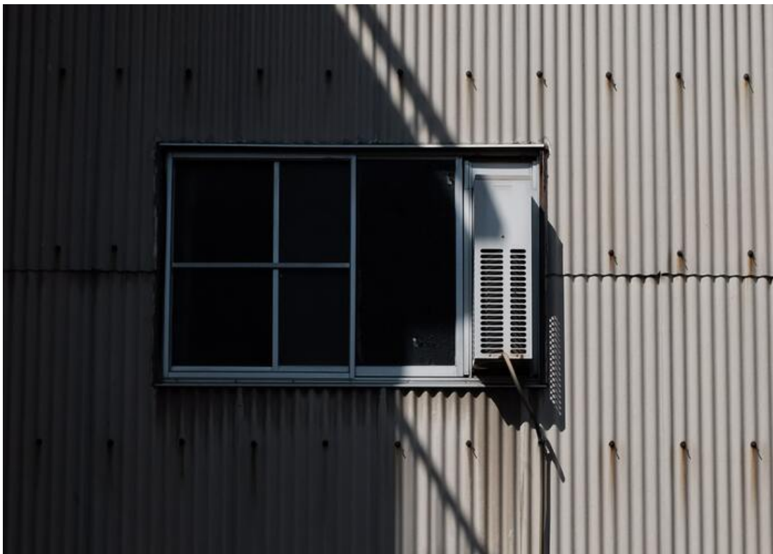
Figure 2. An exterior air-conditioning unit. Source: Mak/Unsplash
