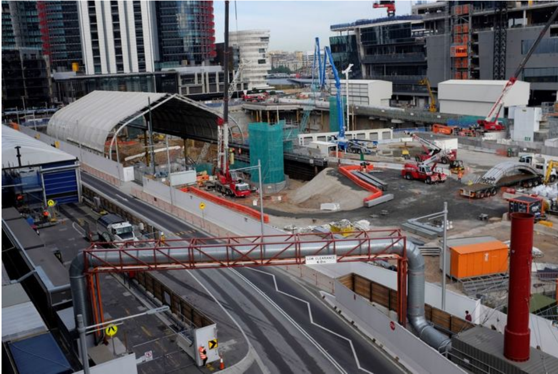
Figure 7. Hickson Road cut through the site of the gasworks and now provides a dividing line for the Western side of the site (right), which was decontaminated by late 2018, and the Eastern side (left), which is still undergoing remediation. Image courtesy of the author.
